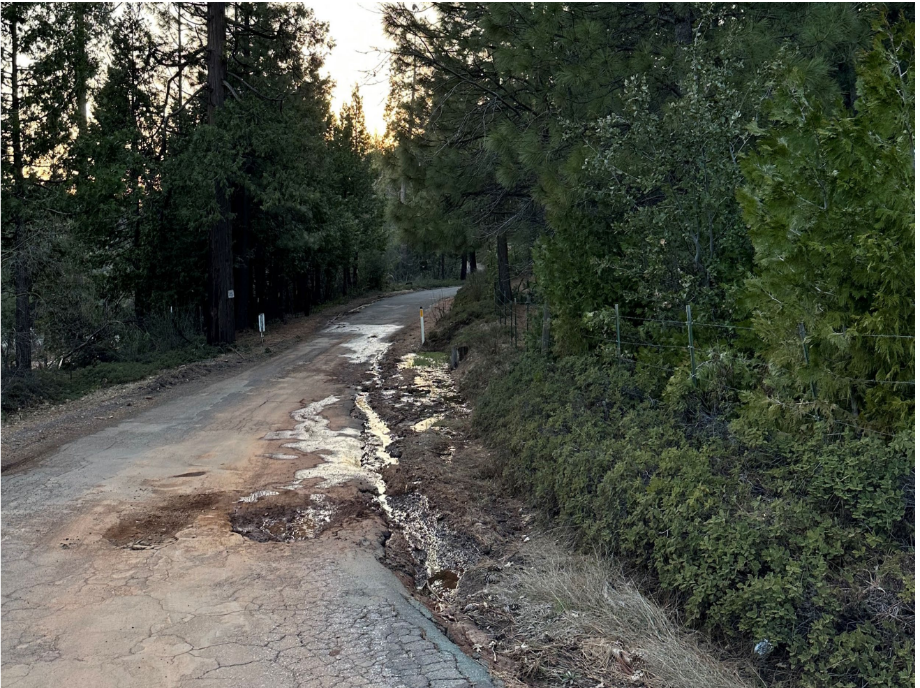
Figure 5.2 Photo of Sheep Ranch Road with washout March 2023
